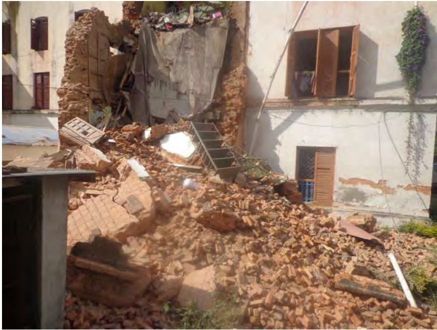
Main building damaged by earthquake
